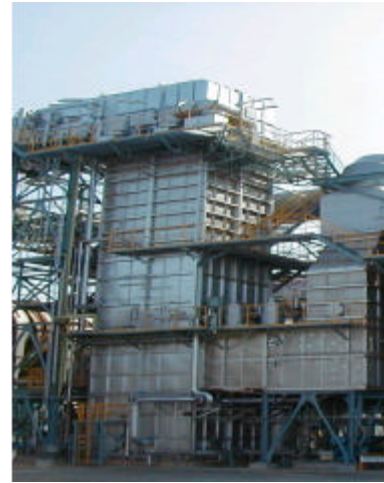
Fig. 13 Outside View of Commercially Operated MDDS
